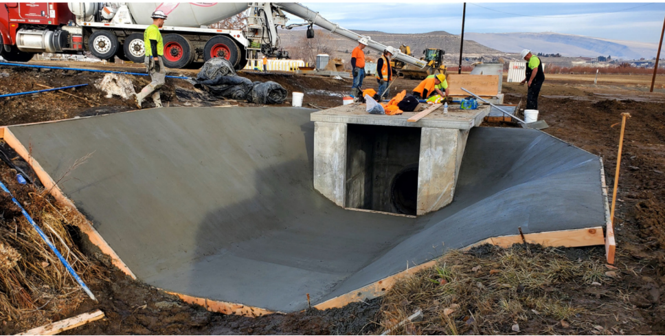
Patrolmen and Tapani, Inc. crews pouring concrete transition from No. 3 Lateral canal
