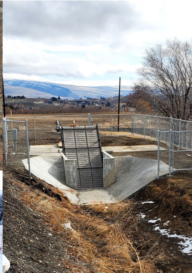
Automated screen from No. 3 Lateral canal to new Guinan Road pipe crossing
