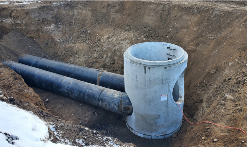
Manhole to 33 and 36-inch pipes crossing Guinan Road
