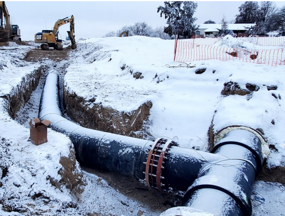
33-inch pipe connecting to existing 36-inch pulled through wood stave siphon in 1987
